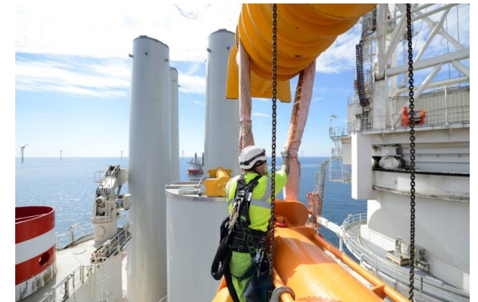
Leading installation company with ~900 employees
